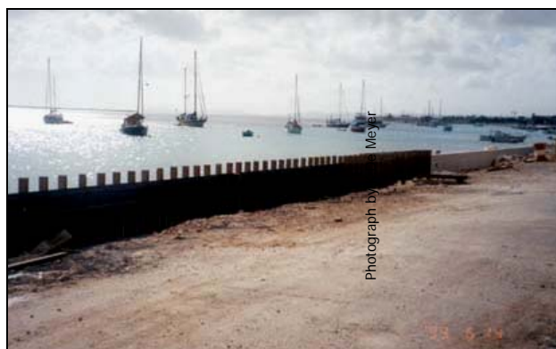
Screening of construction work prevents sediments and debris from entering the sea
